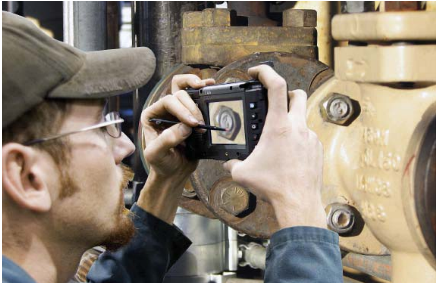
PERMANENT RECORD: A technician uses the camera to document corrosion.
