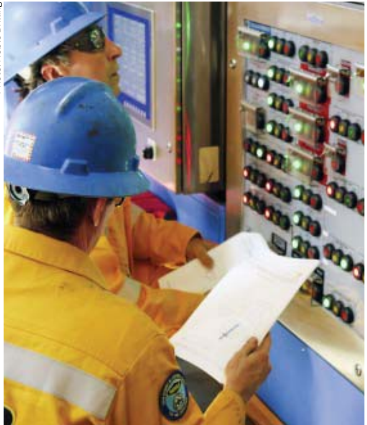
SYSTEMS CHECK: Noble Drilling technicians use live-streaming technology to collaborate with shore while reviewing blowout preventor test procedures in the Gulf of Mexico.
